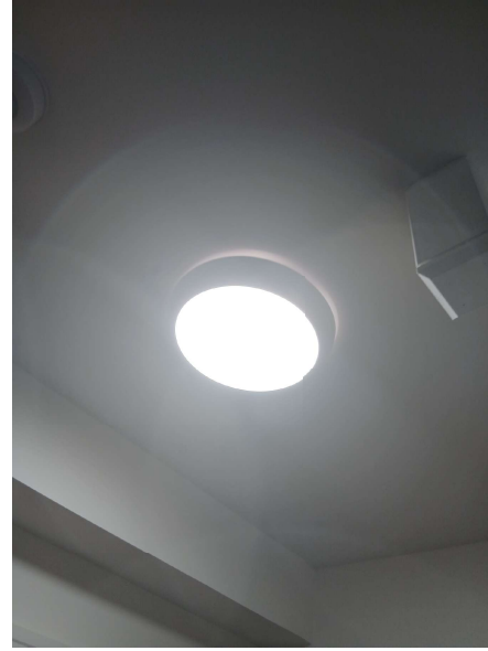
Lighting (Standard and Emergency Lights)
